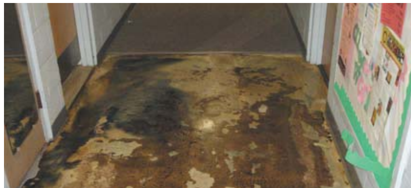
Mold grows in Dyer Hall after a pipe burst and leaked water under the carpet. The prevalence of mold throughout the six dorms in Kissam Quad is attributed to the poor ventilation and air circulation.
