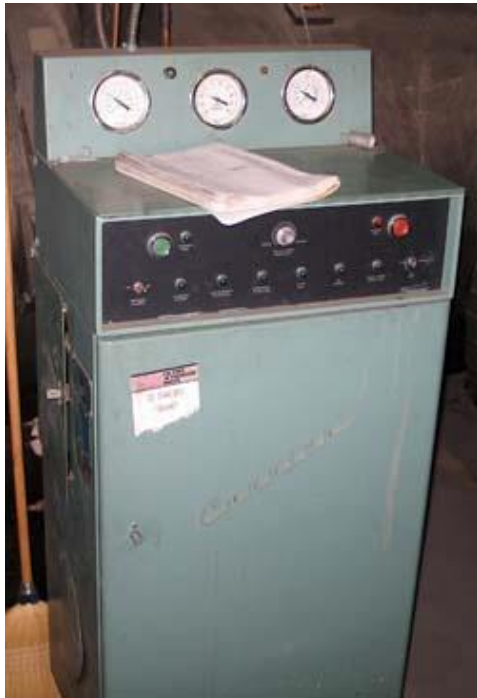
Figure 10: Carrier's Control Panel
