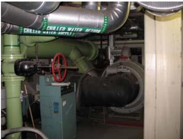
Figure 7: Carrier's chilled water pipes
