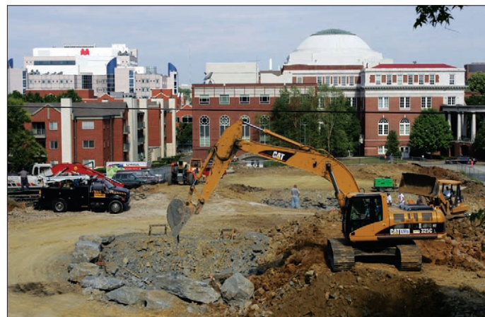
Construction started this spring on The Commons, the first phase of College Halls at Vanderbilt. Five new residence halls will be built on the Peabody Campus where Garrison Apartments, Married Student Apartments and the Peabody Student Center previously stood. The other five existing dormitories will undergo renovations. The ten residence halls, to be known as "houses," will house all first-year students at the University and are scheduled to open fall 2008.
