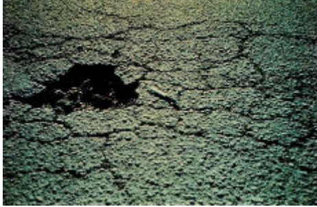
Figure 4. Pothole from Fatigue Cracking (Washington 2005)
