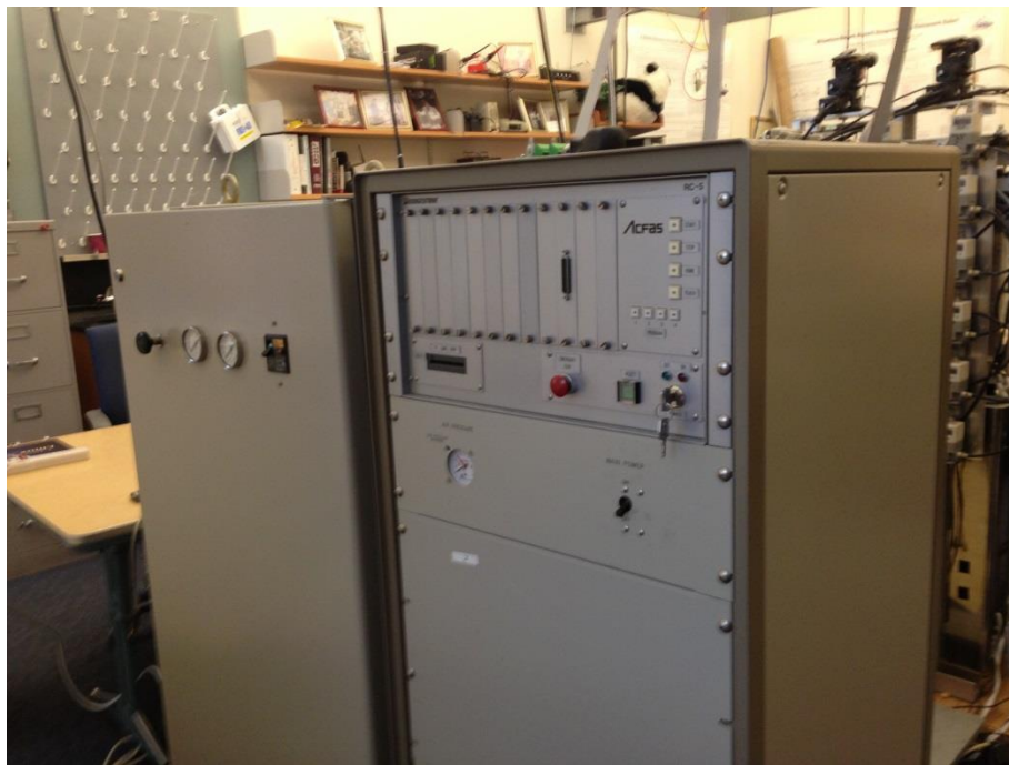
Figure 287 Electrical Control Cabinet
