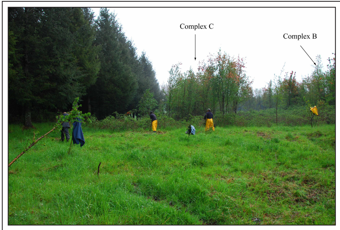
Figure 33: View of workers clearing brush from surface of Santa Sylvania with Complexes C and B noted, looking south.
