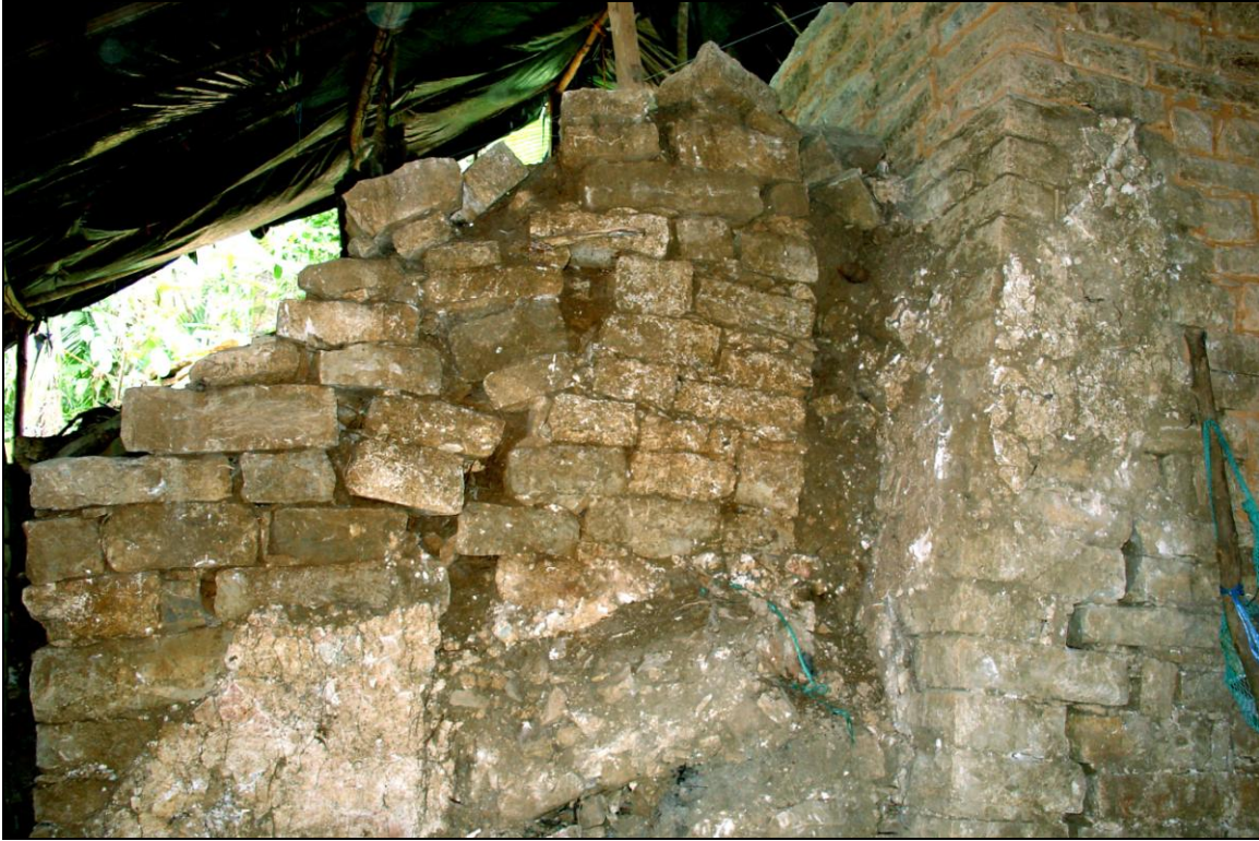
Figure 9.54 Division wall between rooms 7 & 8 with plastered surfaces (Photo by R. Larios, VCAP)
