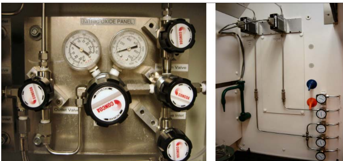
Figure A.8: Left: custom-built regulator panel for hazardous gases. Right: selection bellow valves, in-line filters, and mass-flow controllers.
