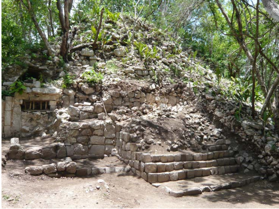
Figure 5.22: Front (south) façade of Palace after conversion to a pyramid during the Terminal Classic period (courtesy of BRAP)
