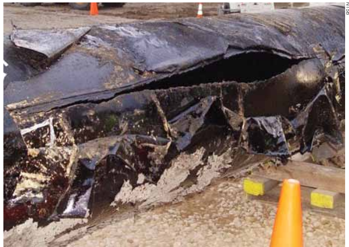
Pipes made of modern composite materials might prevent pipeline ruptures such as this one in Michigan.
