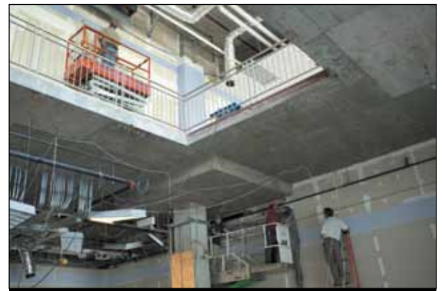
Workers prepare the old Borders location for a new Vanderbilt bookstore, to be operated by Barnes and Noble. The new location is expected to open in October 2011.
