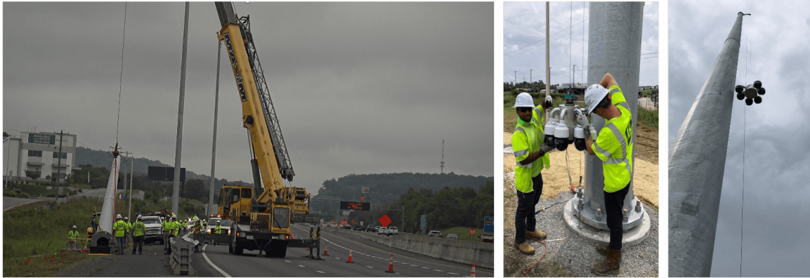
Figure 3.8: Validation system construction. Left: 110-foot poles are raised adjacent to the freeway; middle: Multi-camera mount holds 6 4K PTZ cameras; right: cameras are elevated to the top of the pole.
