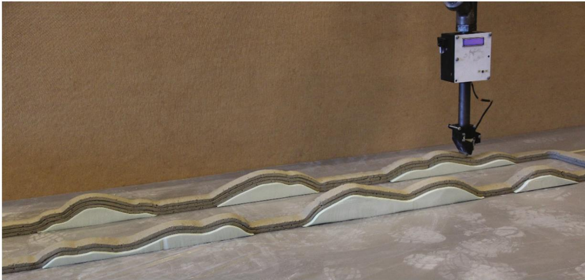
Figure 8 - 3D printing concrete on a non-flat surface with arbitrary curvature and height variations. Adapted from [19].
