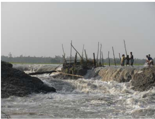
Figure 12. Photo (Laura Benneyworth, 10/19/12). Embankment breach between a rice paddy and tidal channel (Nalian River). Photo taken from boat on Nalian River during low tide looking towards Polder 32.
