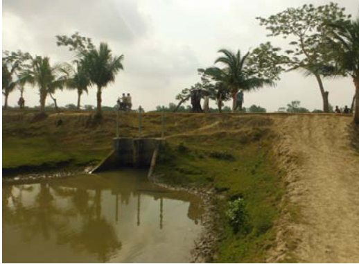
Figure 11. Photo (5/19/12). A sluice gate constructed through Polder 32 embankment. Photo taken from inside of Polder 32 looking towards Nalian River beyond embankment.
