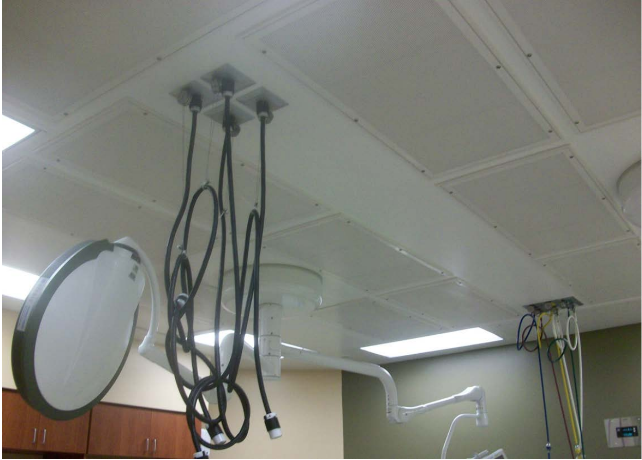
Figure 3 – The operating rooms in this study used ceiling mounted supply diffusers providing conditioned and filtered air over the surgical area. Ceiling mounted equipment, such as booms and lights, can impact the flow of air and location of diffusers.
