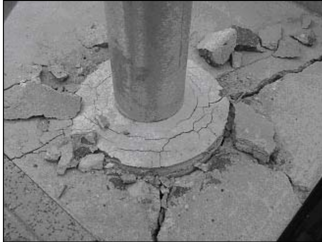
Figure 14: Expansion due to sulfate attack
