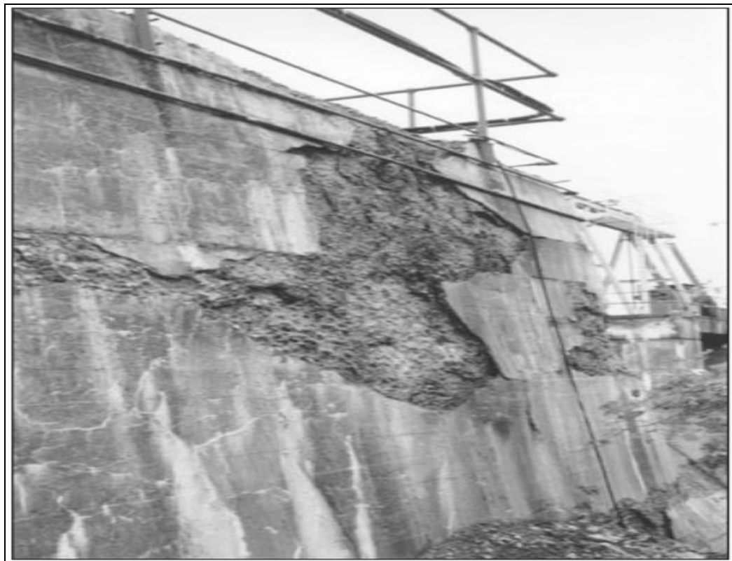
Figure 15: Damage from freeze-thaw cycle
