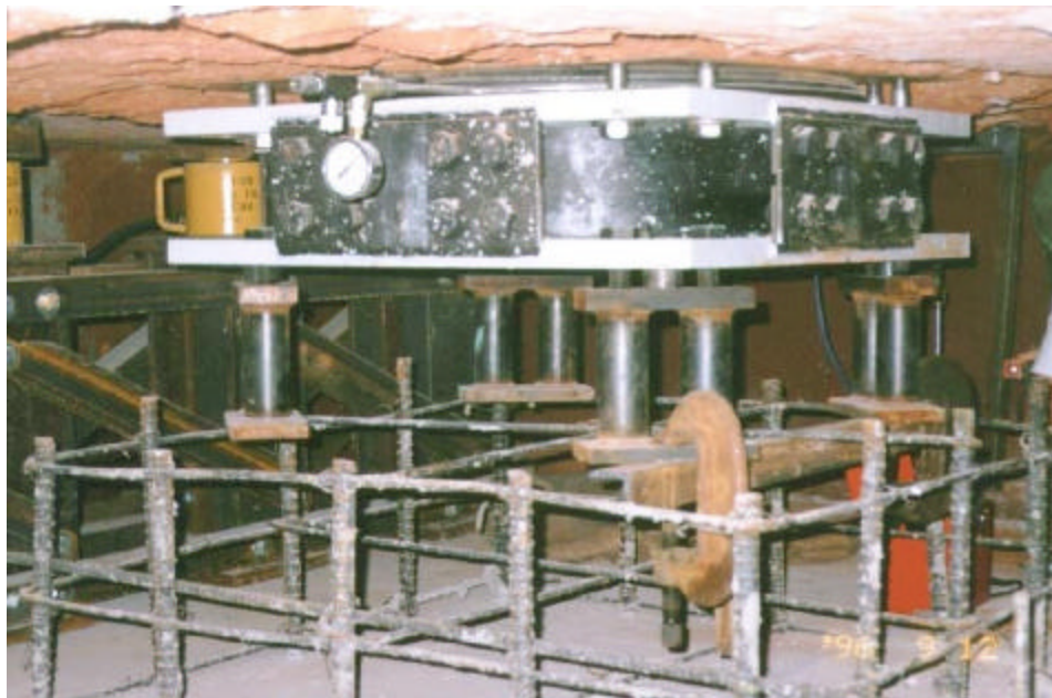
Figure 8. Base isolation system used under State House, Columbia, South Carolina
